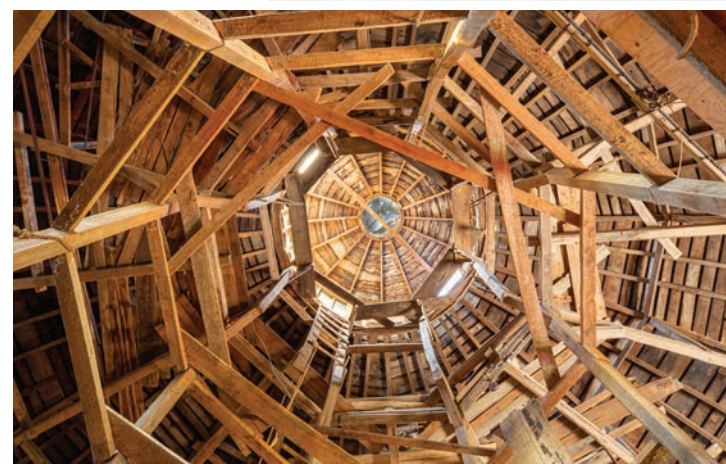
View looking up the center of the barn in the space originally held by a redwood silo. Photo by Dave Austin
