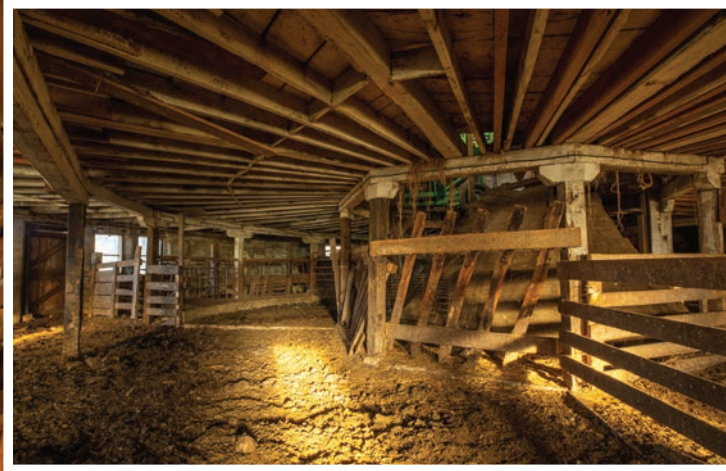
A view of the first level before restoration showing the flooring joists supported by the ring beams. Photo by Dave Austin
