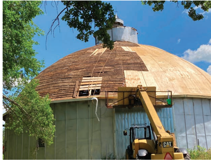
The roof replacement required over 120 4x8 sheets of plywood sheathing. Photo by Kari Friedlein
