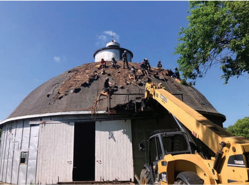
Roofers tackling the challenging job of removing the old shingles. Photo by Kari Friedlein
