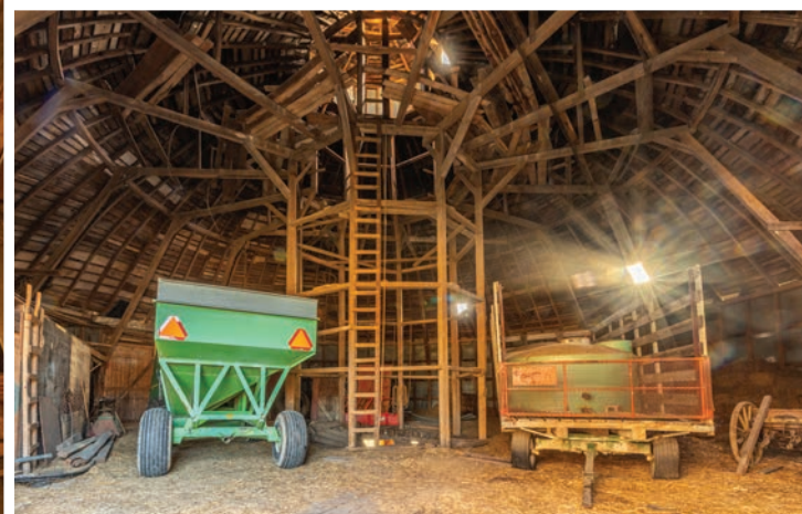
A view of the second level showing the immense size of the 72 foot diameter barn. Photo by Dave Austin
