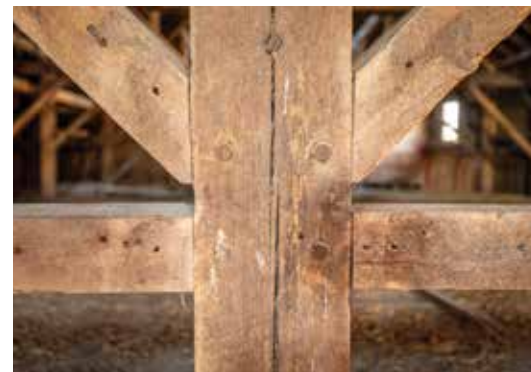
Mortise and tenon joints secured with wood pegs are visible in the haymow.
