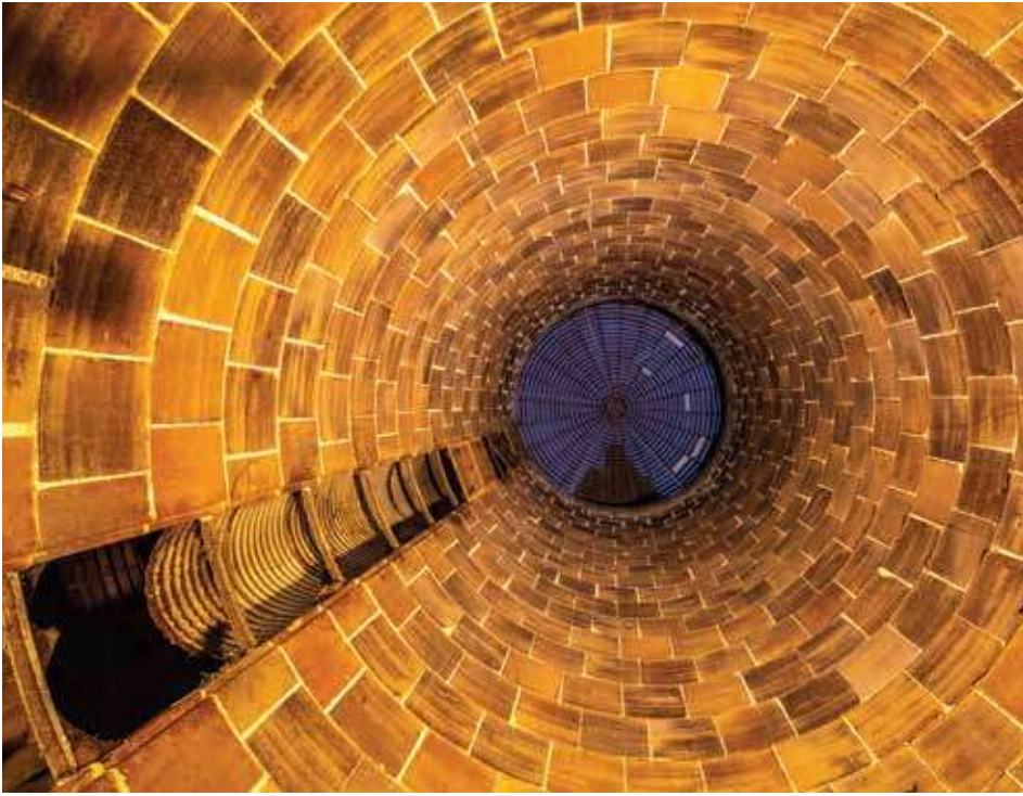
Early morning view looking up through the central clay tile silo when the old roof was removed.
