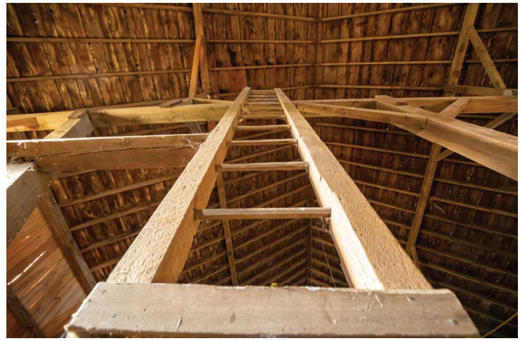
View looking up one of the haymow ladders used to get to the top stored hay when the barn is full.
