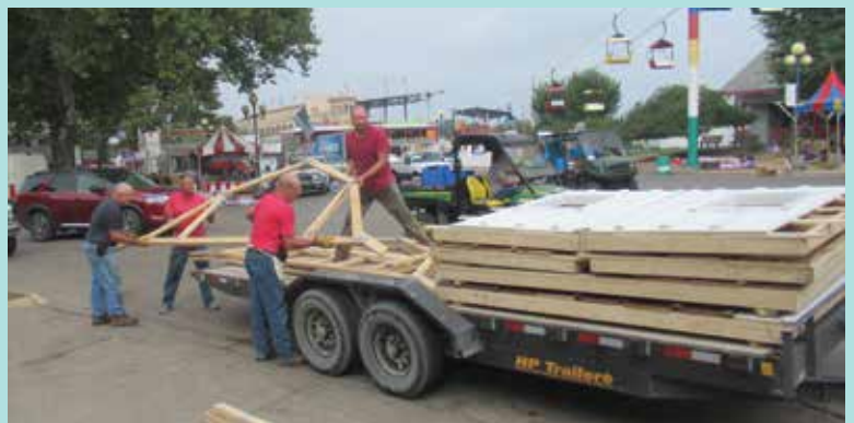
That’s a wrap! After the fair was complete, the barn was taken down and hauled to storage to return in 2024. Left to right: Wayne Frost, Craig Pftantz, Jim Frost, and Ryan Pfantz.
