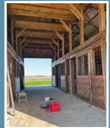
Interior view after pouring of the concrete floor and installation of the stalls.
