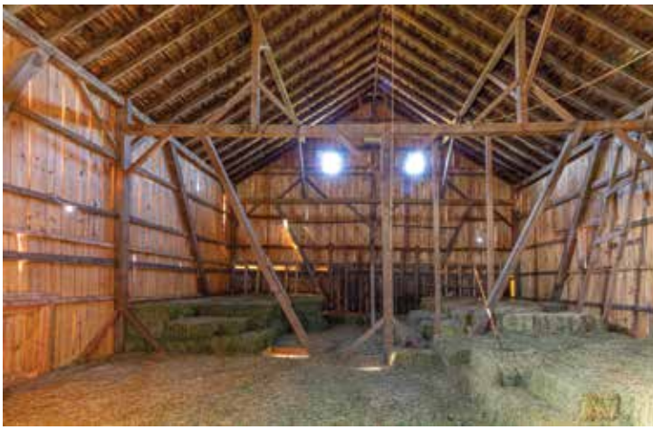
The haymow continues to be used for storage of square bales of hay for Jim's flock of sheep.
