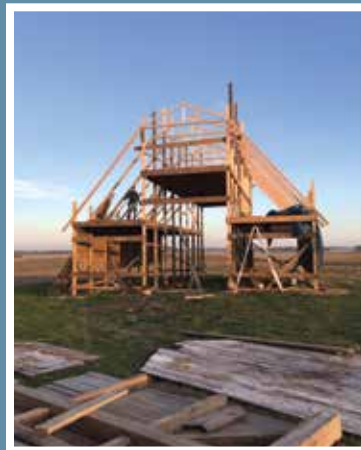
Framing stage at the barn's new location using a combination of new and salvaged wood.
